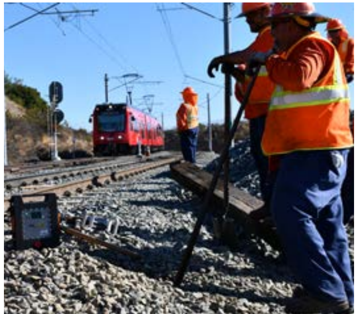
MTS track workers stand clear as a Trolley passes through a work zone. An early warning detection device sits in the foreground.
