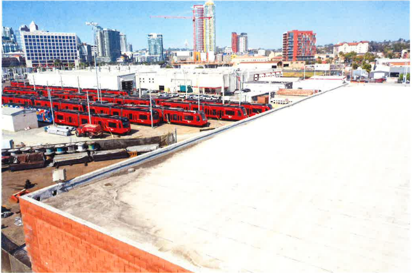
4.1-e Water Ponding on Roof – Northwestern Corner at Roof
