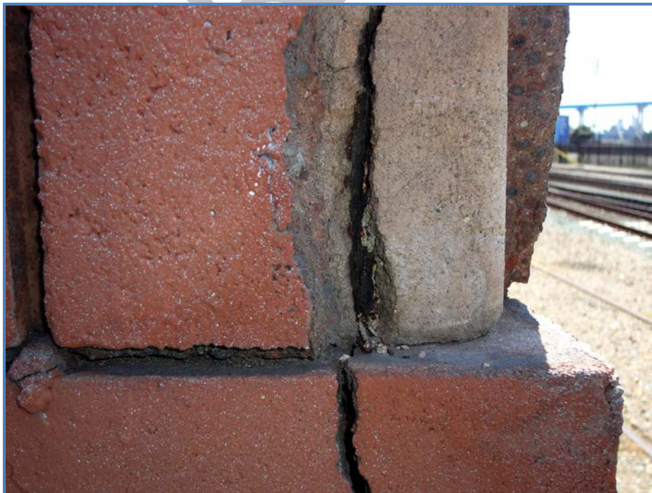
Image 33 – Damaged West Corner
