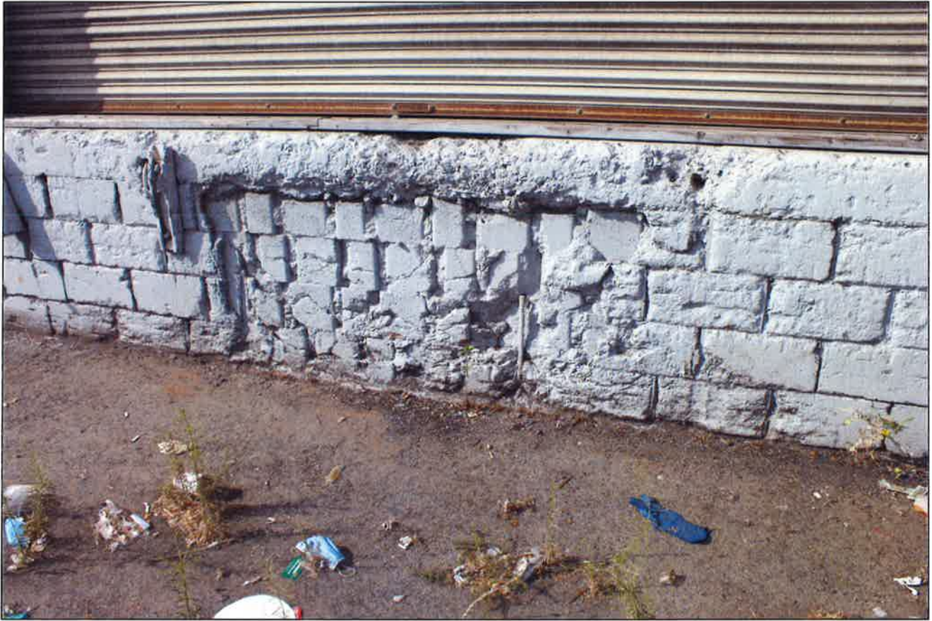
3.2-c Deteriorated/ Patched CMU Blocks – East Elevation
