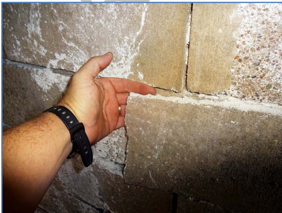
Image 39 – Spalling Block Face
