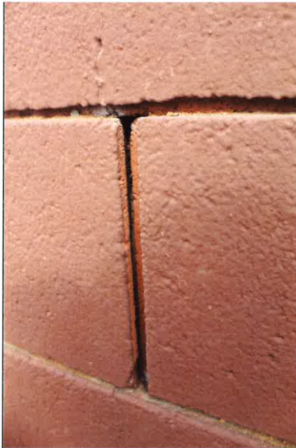
3.1-a Exterior CMU Wall – Open Bead Joints
