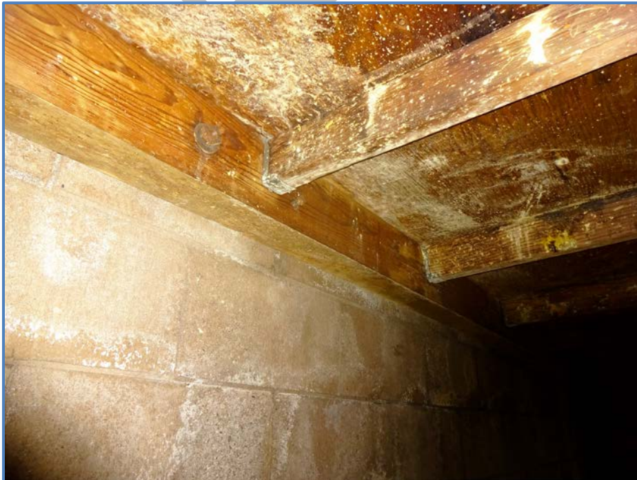
Image 45 – Past Water Damage
