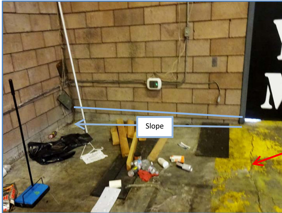
Image 46 – Settled/Cracked Slab at West End
