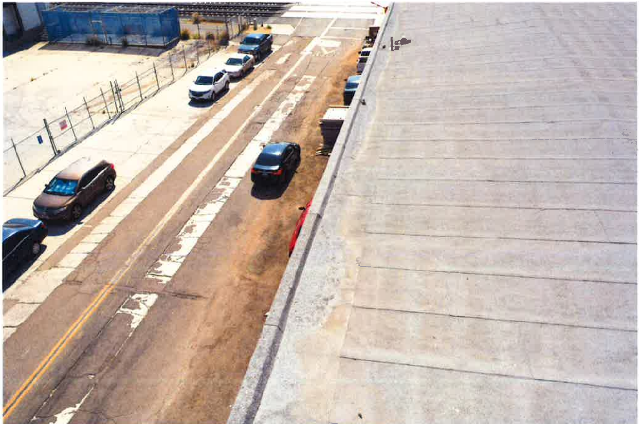
4.1-b Condition of Roof at Southern Edge – Loose Roofing Granules
