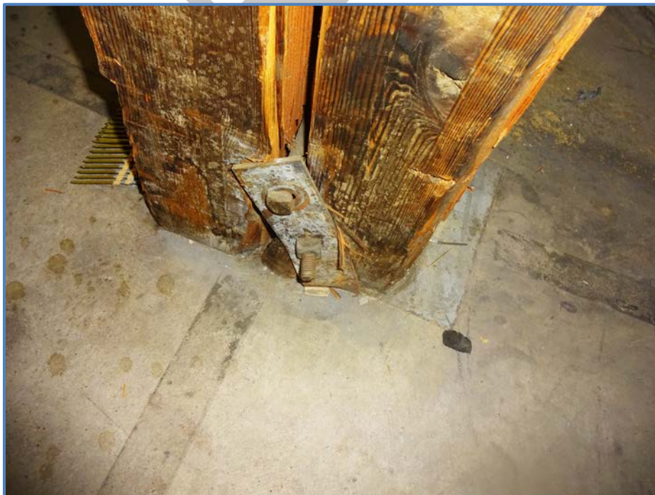
Image 15 – Severe Column Damage
