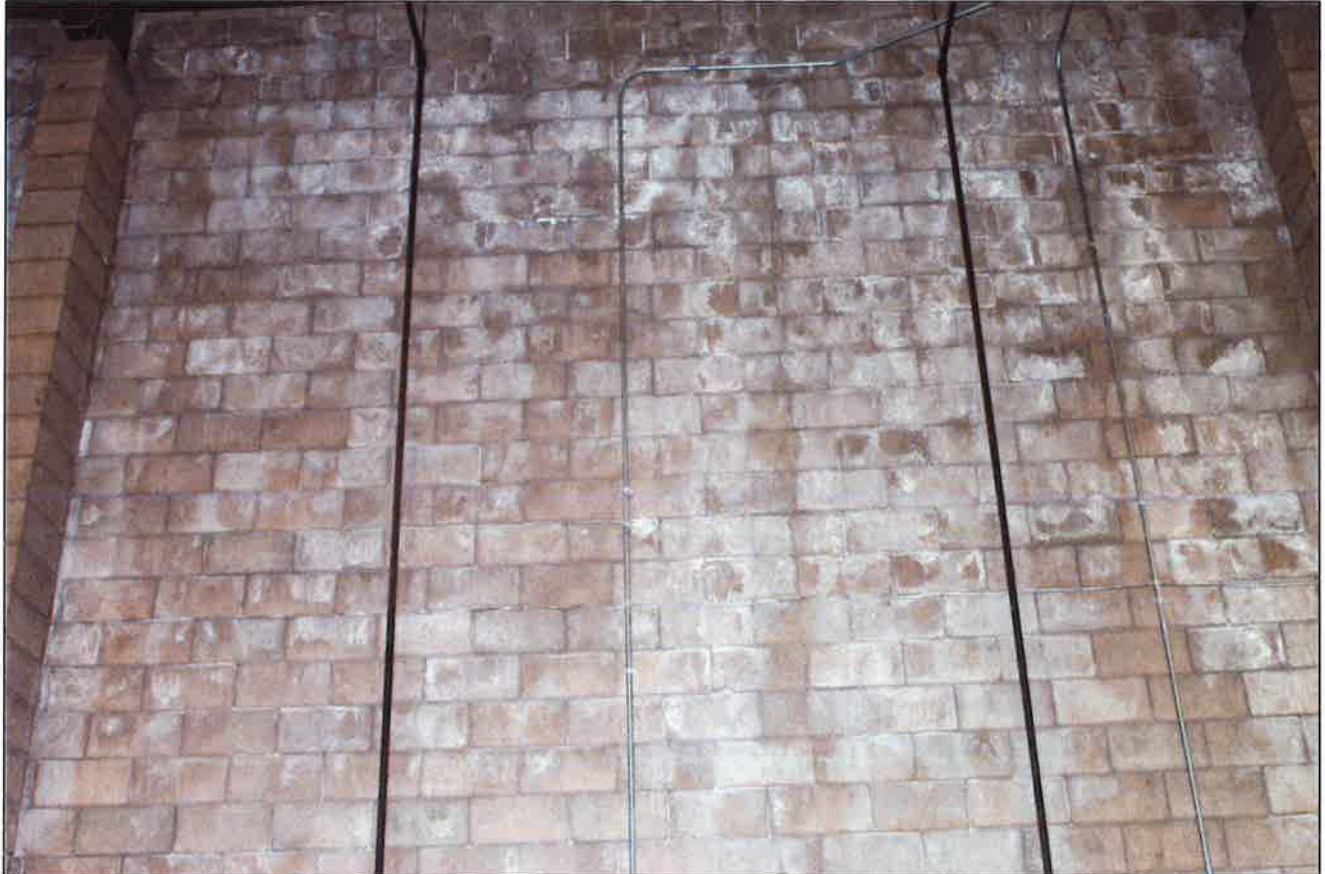
3.3-d Water Stained Exterior Wall
