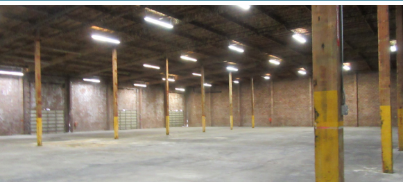
Fire Sprinkler System Evaluation and Egress Requirements
