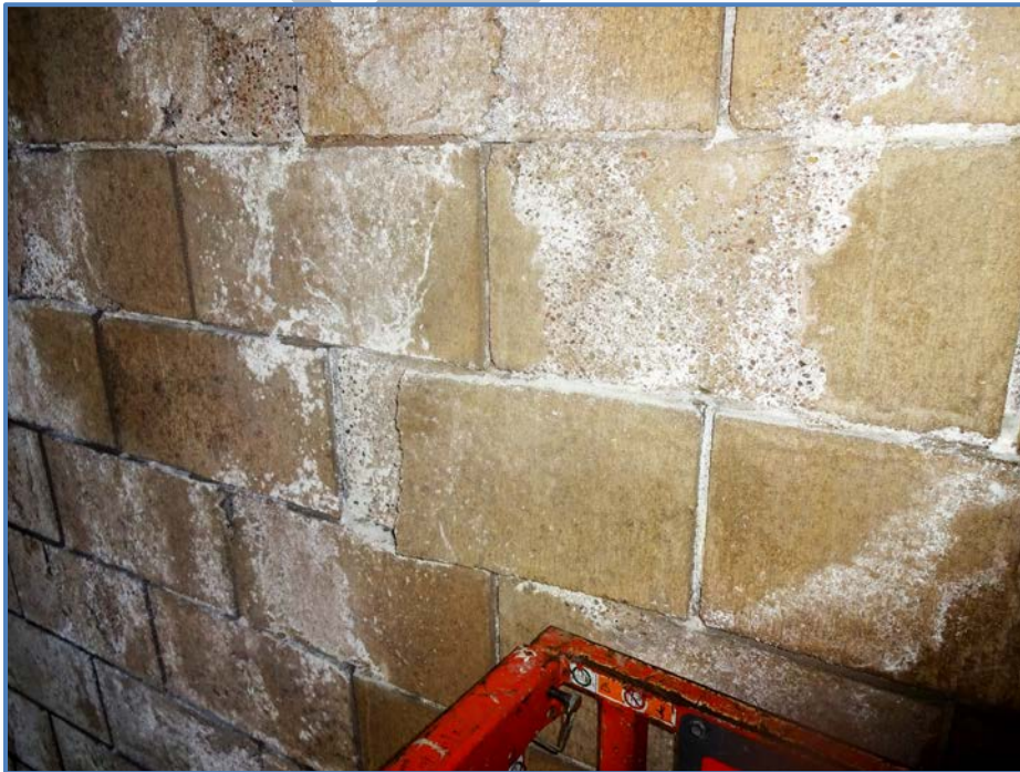
Image 43 – Efflorescence on Walls
