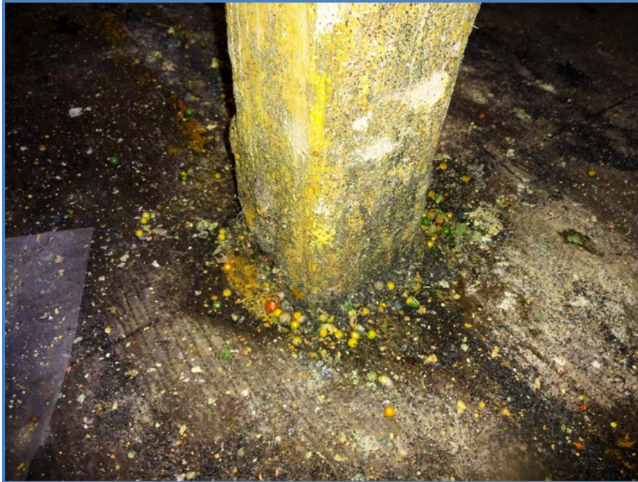
Image 26 – Layer of Material at Column Base
