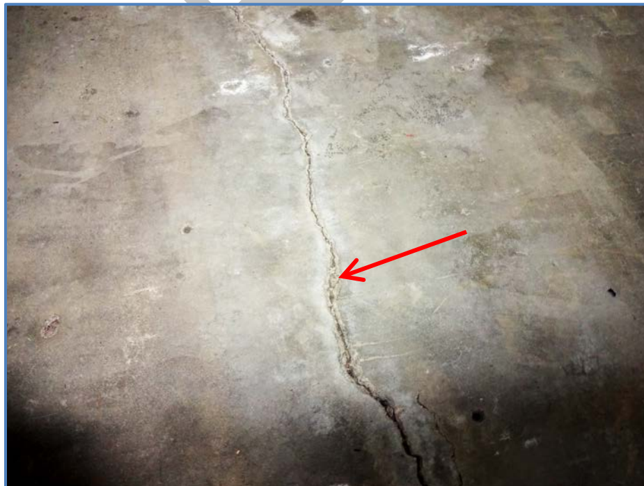
Image 47 – Typical Slab Crack
