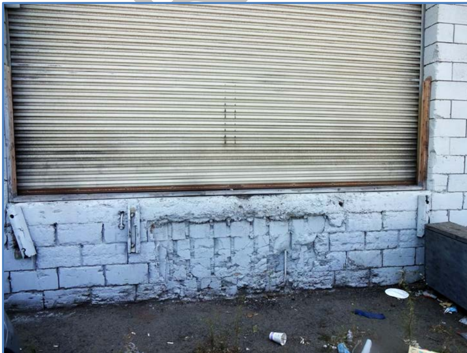
Image 37 – Damage at Loading Dock
