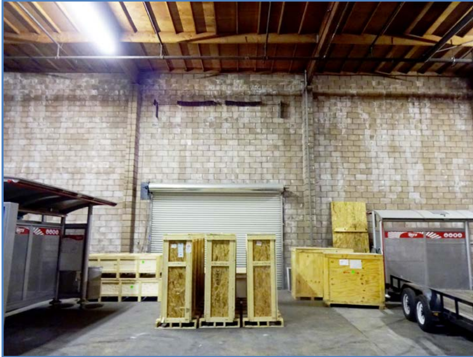
Image 42 – Efflorescence on Walls
