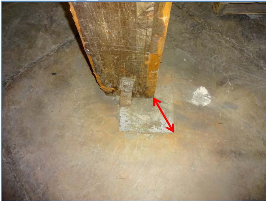
Image 17 – Dislocated Column with Severed Plate
