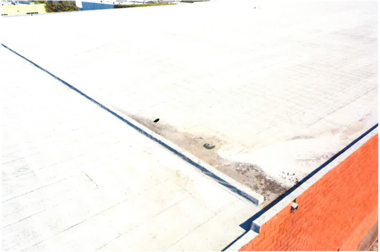
4.1-g Water Ponding at Low Curb/ Roofing Scupper
