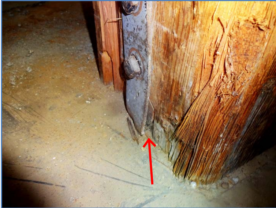
Image 16 – Severed Steel Plate
