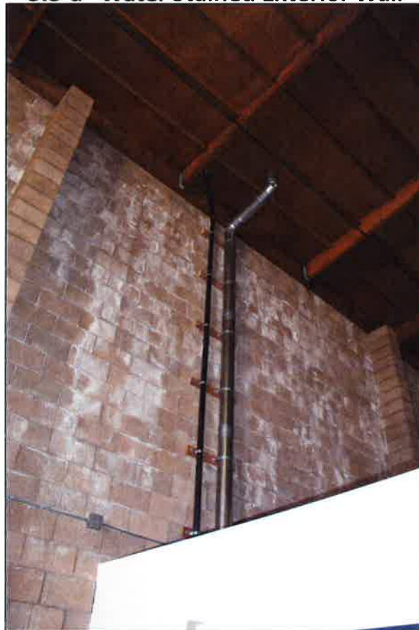
3.3-b Water Stained Exterior Wall
