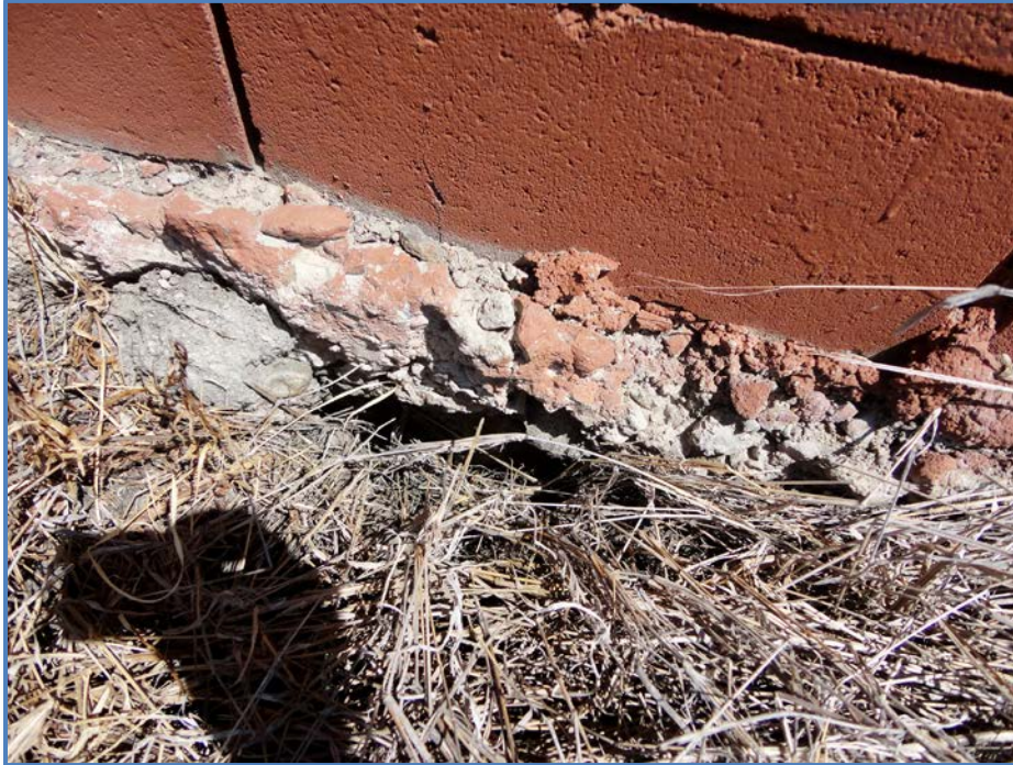
Image 40 – Train Side Undermining
