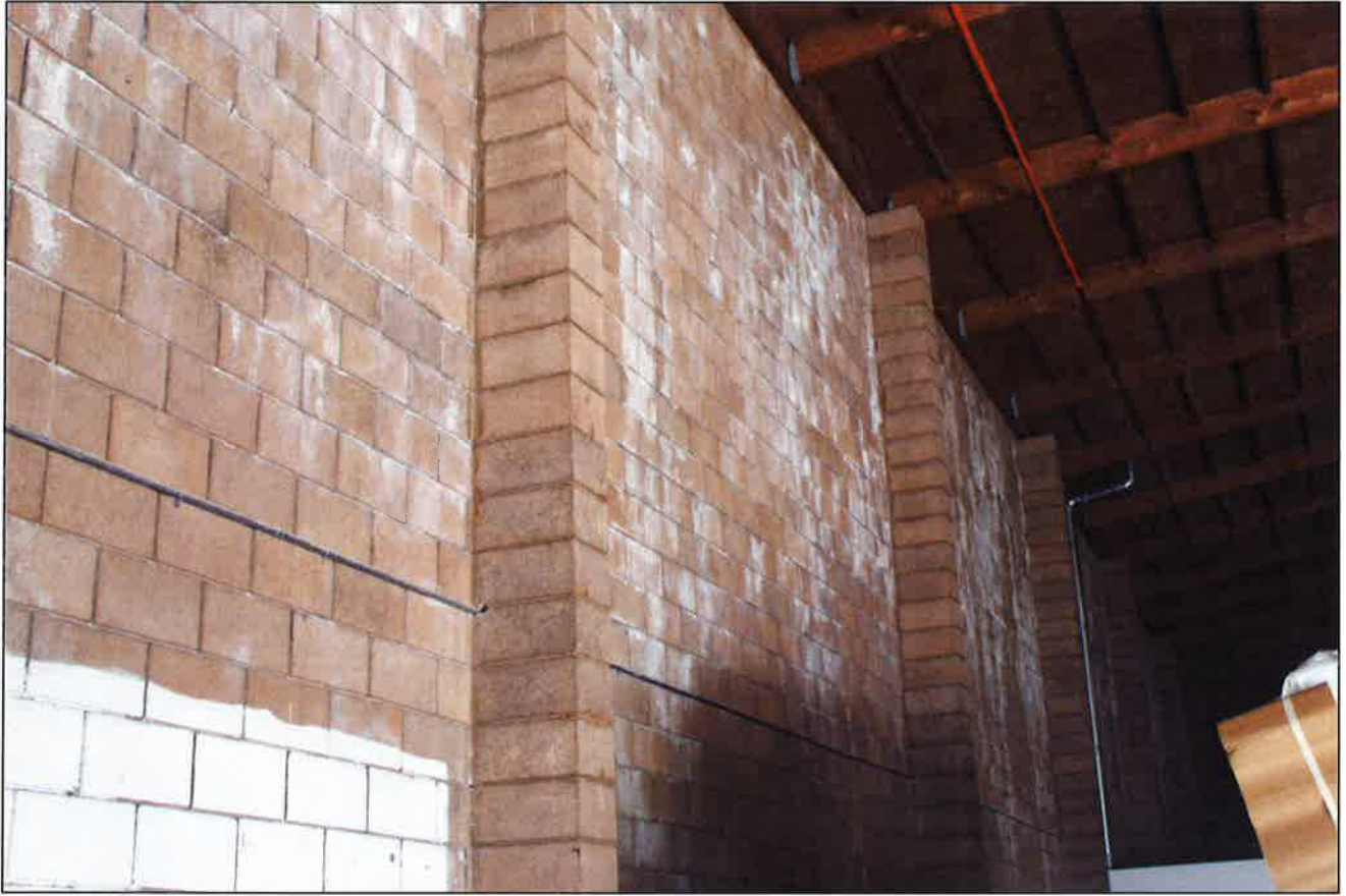
3.3-a Water Stained Exterior Wall
