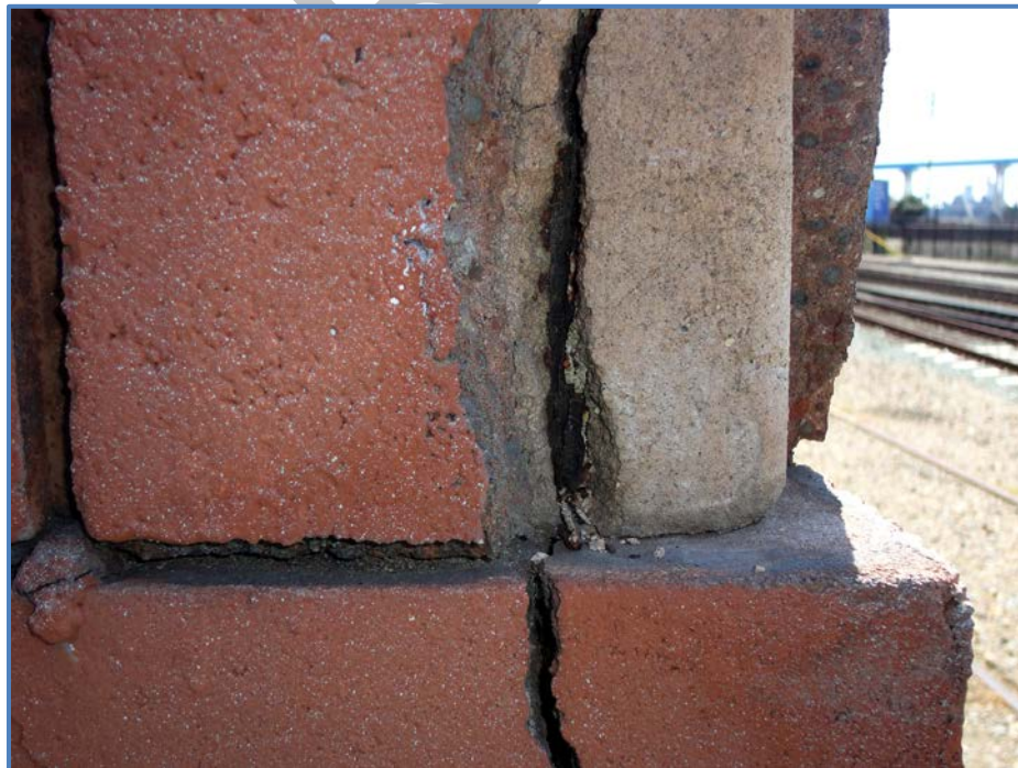
Image 33 – Damaged West Corner
