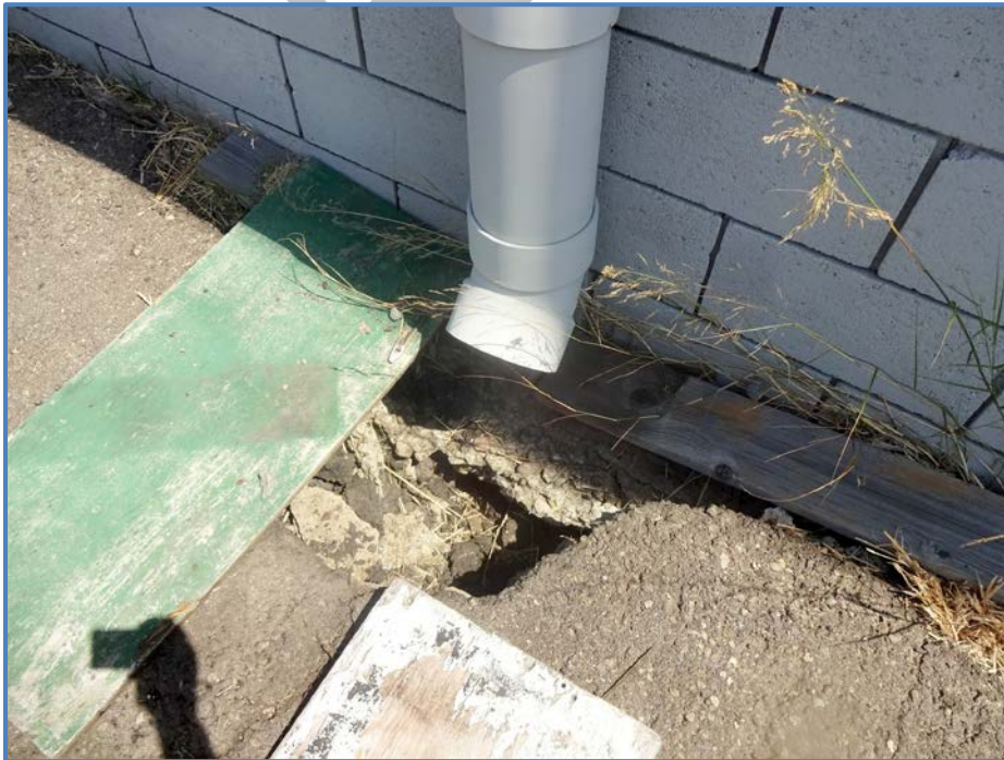
Image 41 – West Parking Lot Undermining
