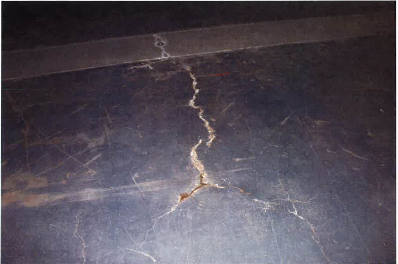
2.3-a Cracks in Concrete Slab
