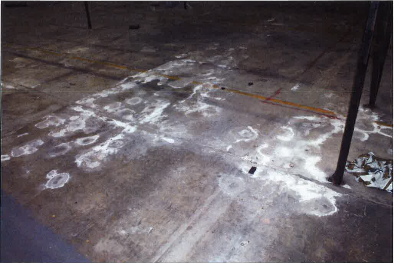
2.4-a Passage of Water Through Concrete Slab - White Efflorescence
