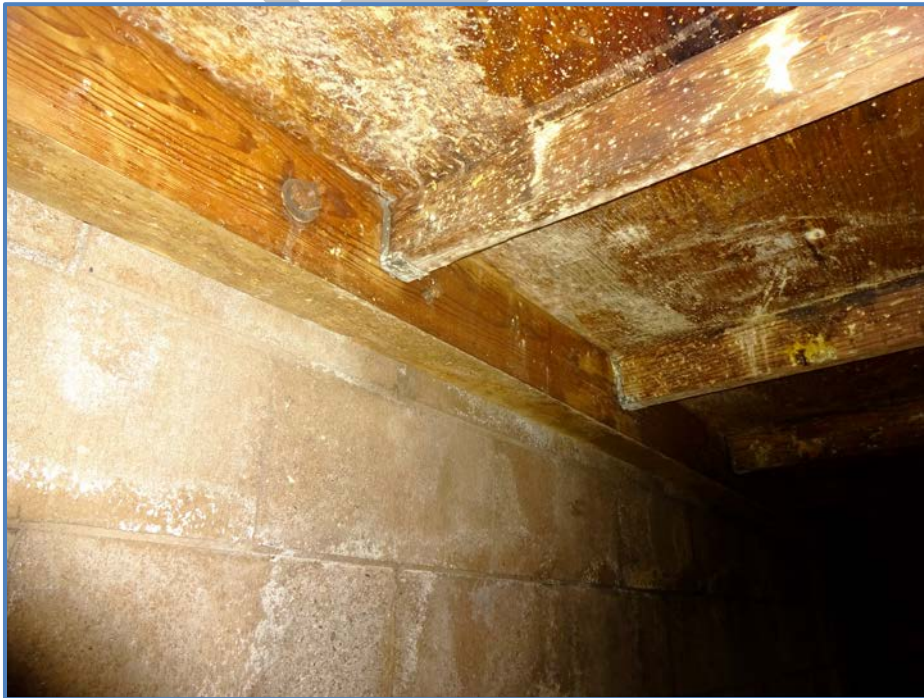
Image 45 – Past Water Damage
