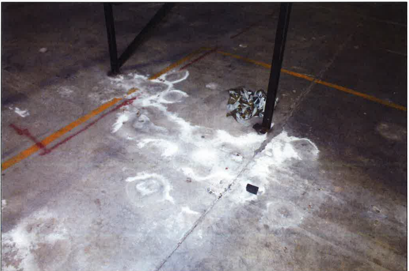
2.4-b Passage of Water Through Concrete Slab – White Efflorescence
