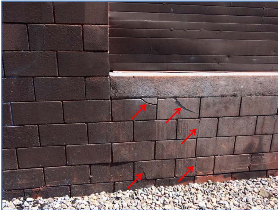
Image 36 – Damage at Loading Dock
