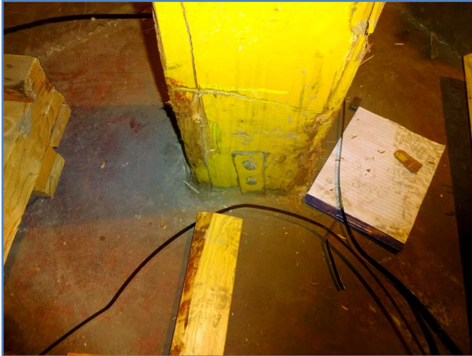
Image 18 – Minor Column Splitting
