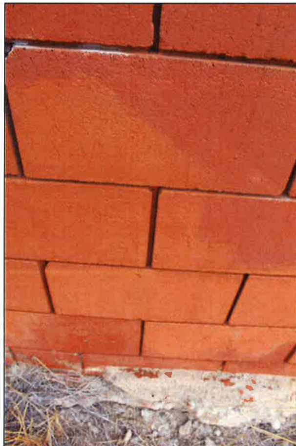
3.1-b Exterior CMU Wall – Open Bead Joints
