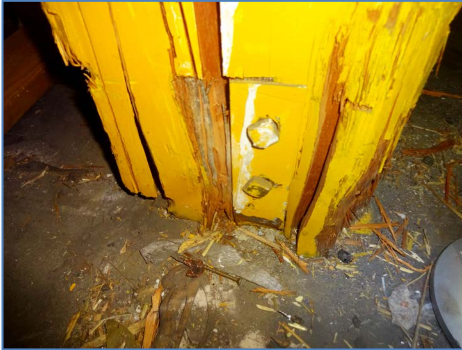
Image 14 – Severe Column Damage
