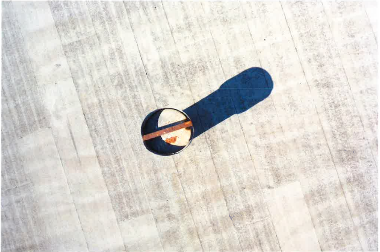
4.1-a Condition of Composition Roof – Missing Granules
