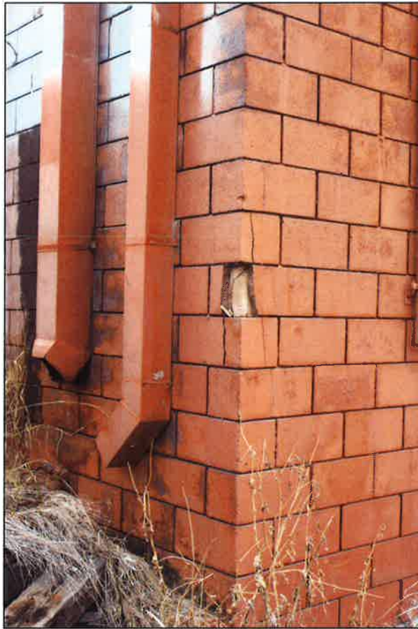
3.2-a Damaged CMU Blocks – Northwest Corner of Building
