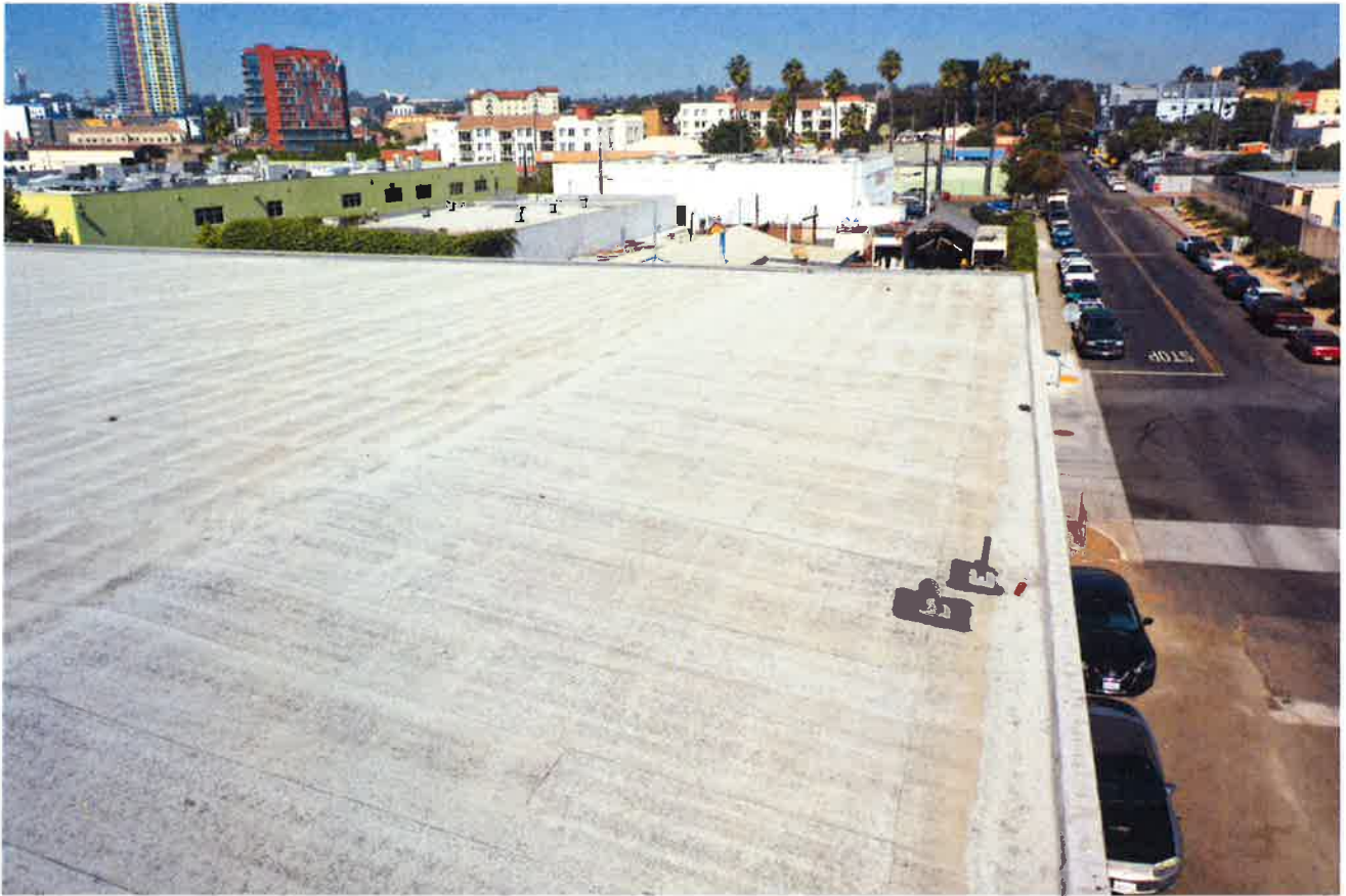
4.1-c Typical Edge Condition – Granular Finish Deposited at Roof Edge/ Drainage Swale
