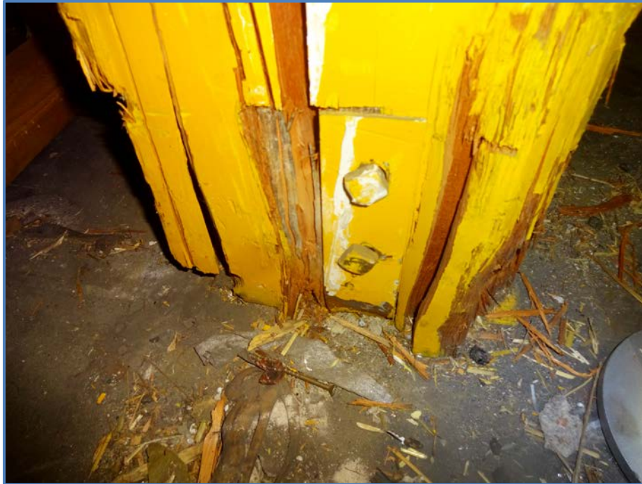
Image 14 – Severe Column Damage
