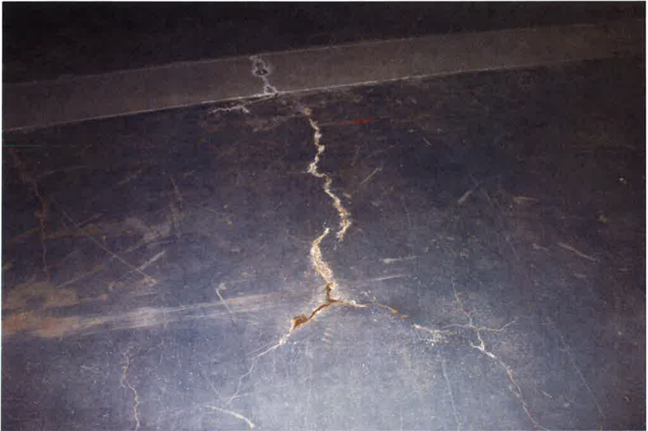
2.3-a Cracks in Concrete Slab
