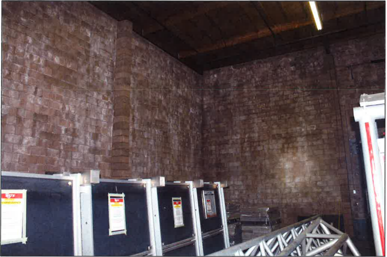
3.3-c Water Stained Exterior Wall
