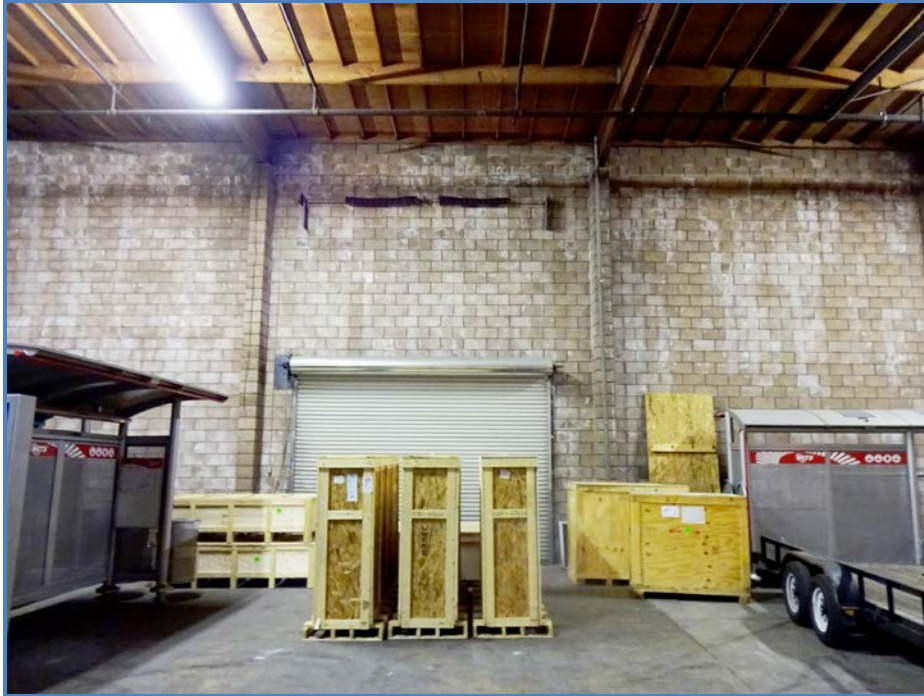
Image 42 – Efflorescence on Walls
