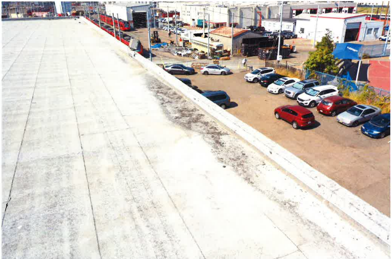
4.1-f Water Ponding on Roof – Eastern Edge of Roof
