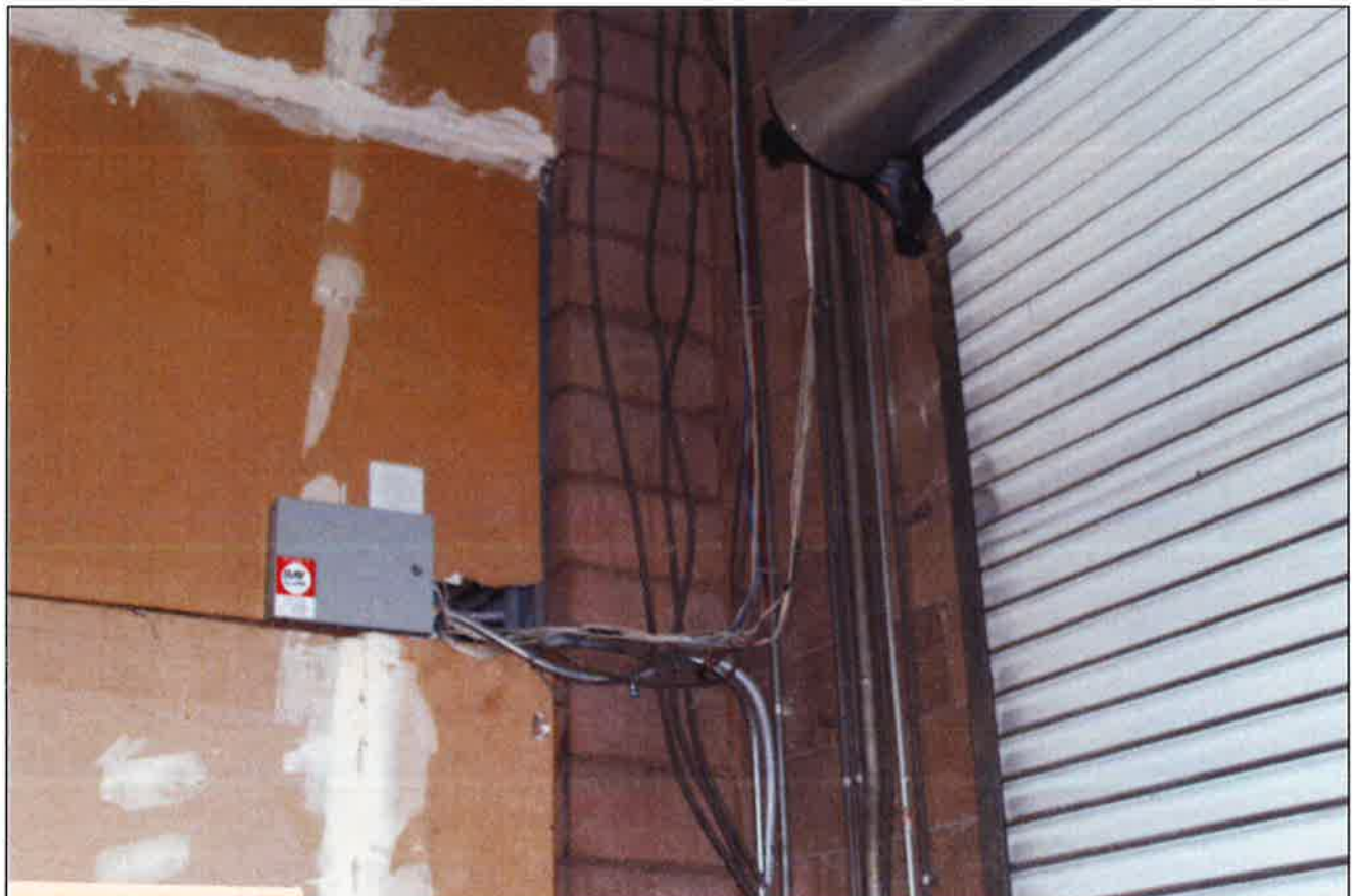
8.0-b Unsealed Electrical Penetrations at Fire Rated Gypsum Board Wall
