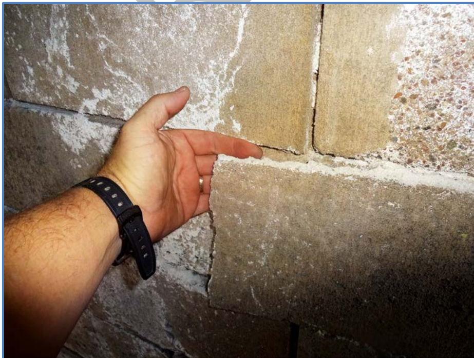
Image 39 – Spalling Block Face
