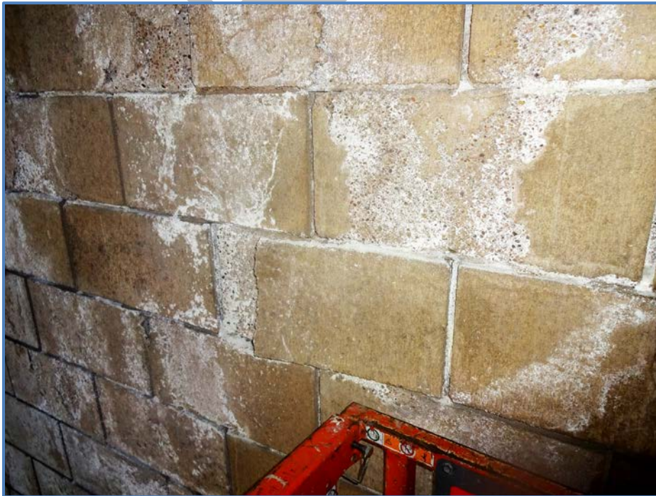
Image 43 – Efflorescence on Walls
