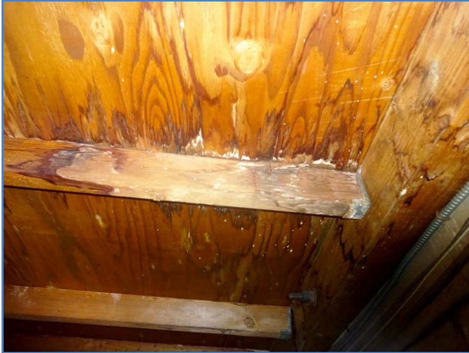
Image 44 – Past Water Damage
