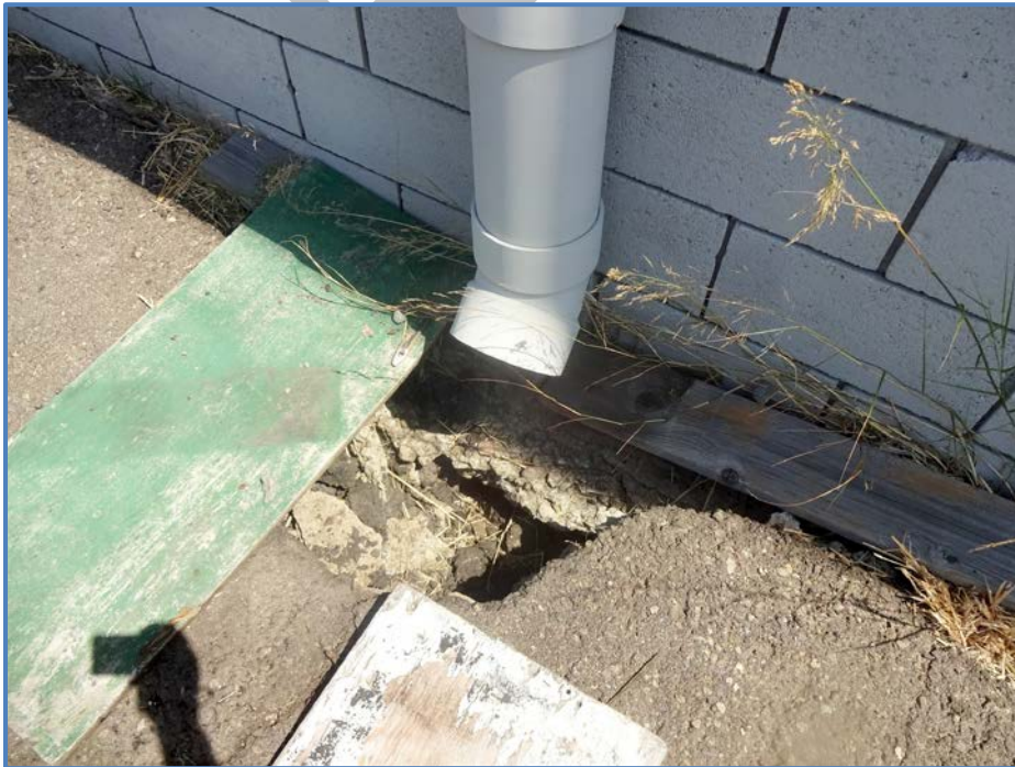
Image 41 – West Parking Lot Undermining
