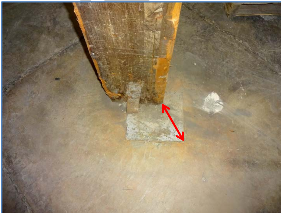
Image 17 – Dislocated Column with Severed Plate
