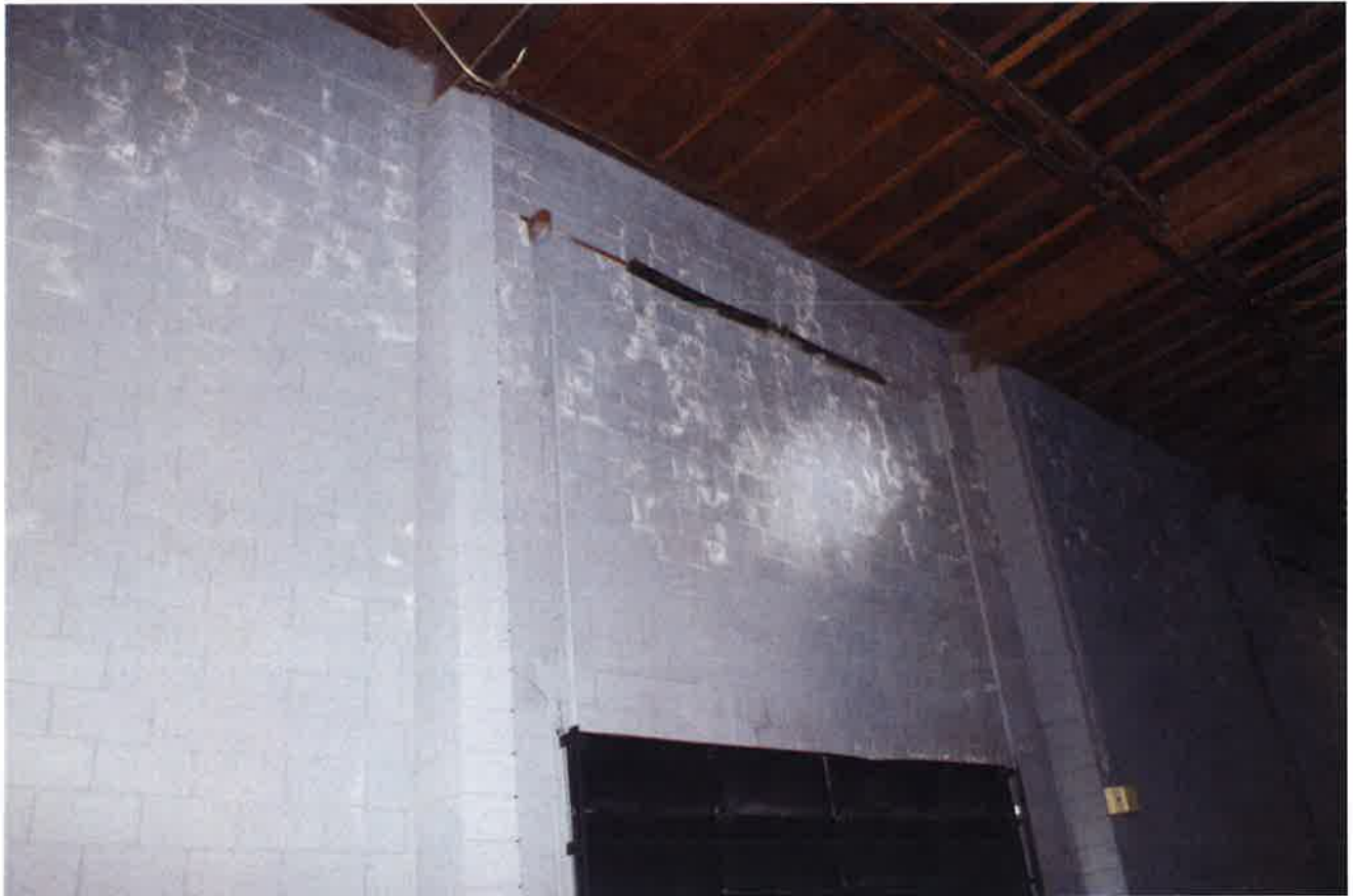
3.3-e Water Stained Exterior Wall – Through Painted Surfaces
