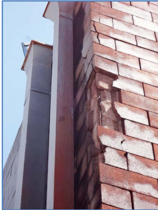
Image 32 – Damaged West Corner
