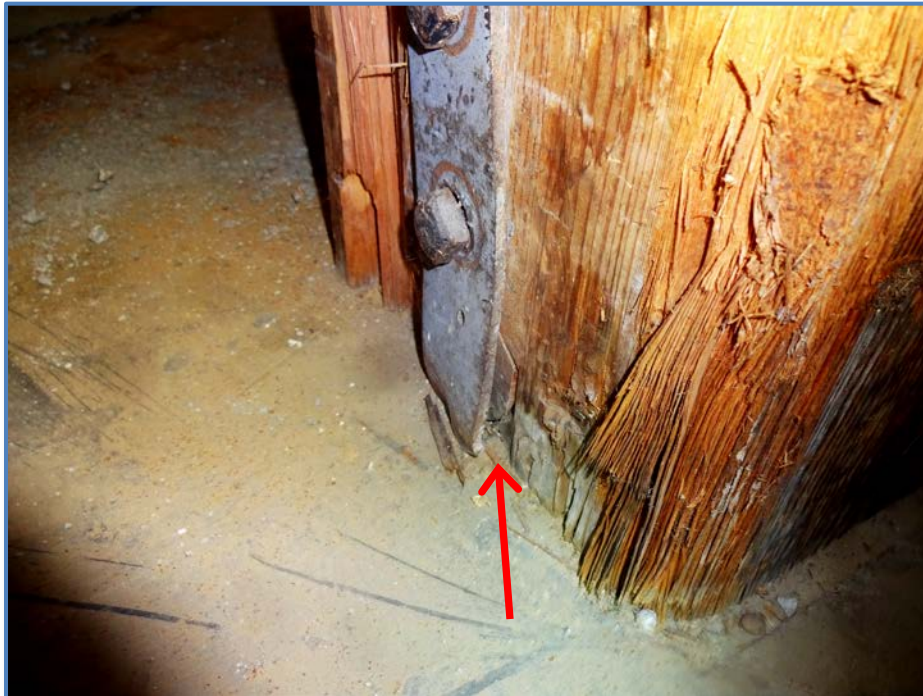
Image 16 – Severed Steel Plate
