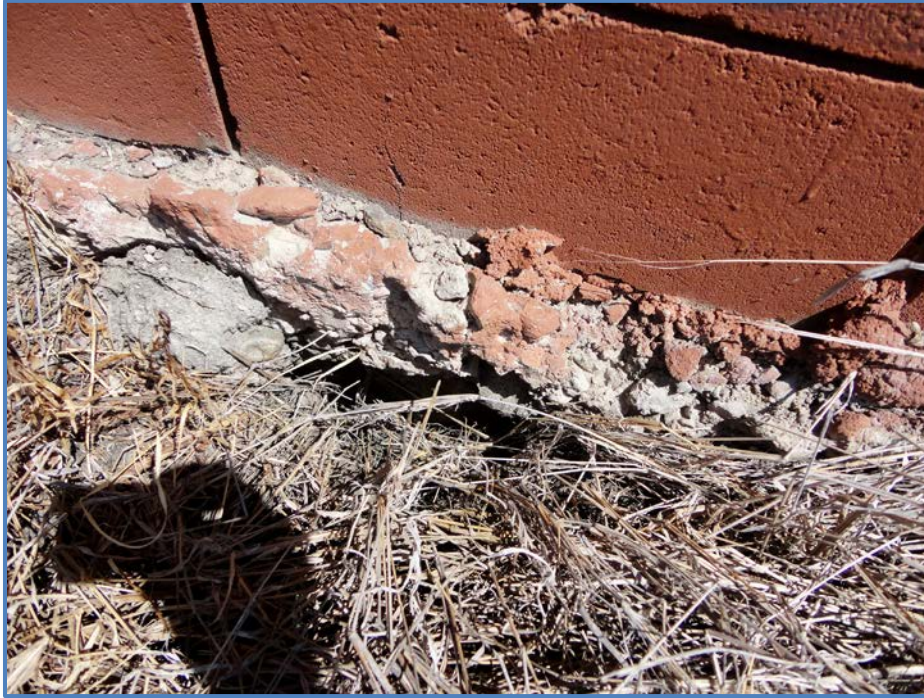
Image 40 – Train Side Undermining
