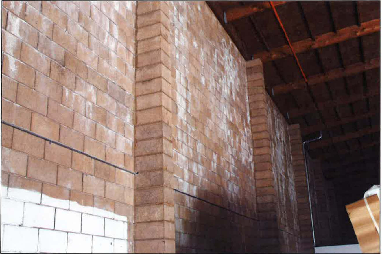
3.3-a Water Stained Exterior Wall
