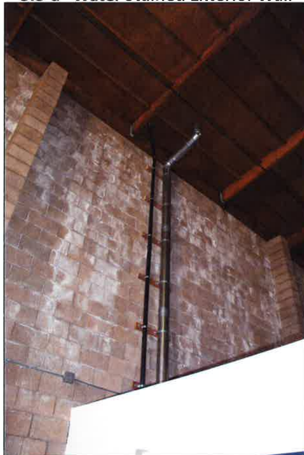
3.3-b Water Stained Exterior Wall
