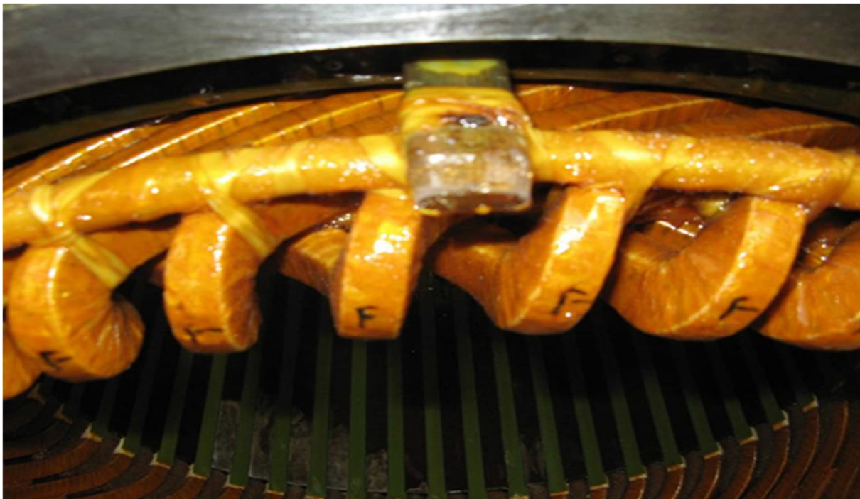
Figure 5 - Motor windings tied to stator housing by Siemens LD
