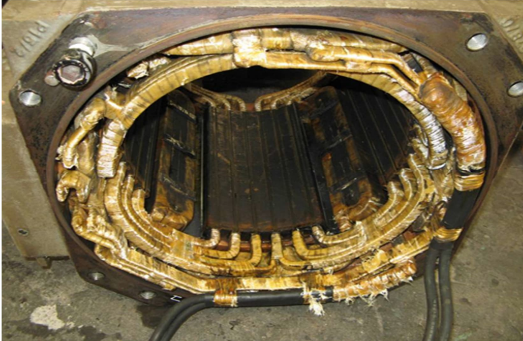
Figure 3 - Motor cleaned with improper chemicals
